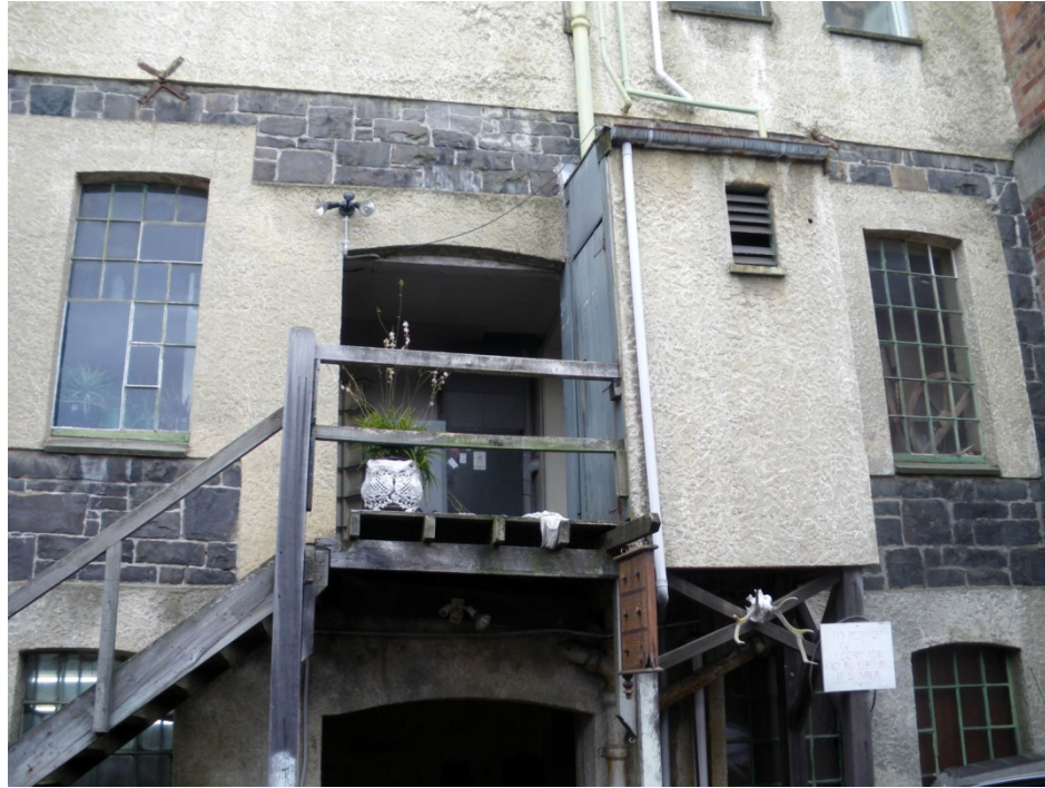
The back of 403 Princes St with a shingle above the doorway to Anderson and Paul's basement workshop (2010).
