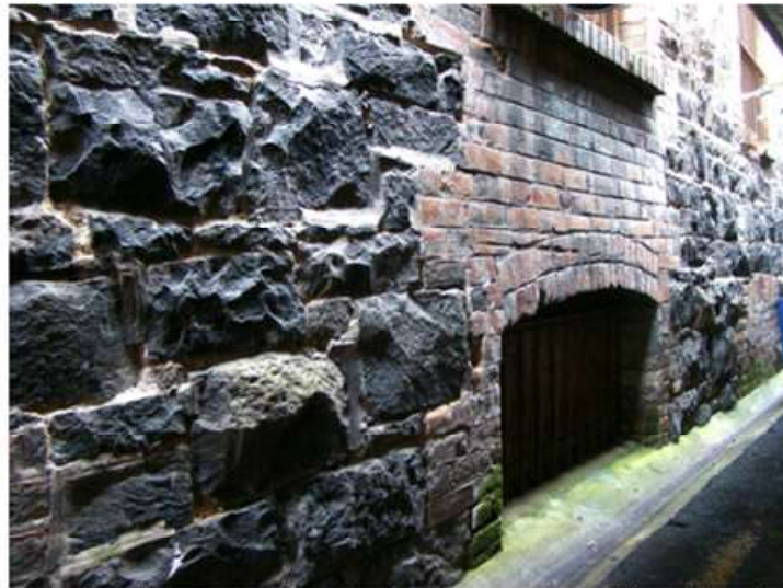
19. Detail, Blacket Lane, December 2012. Photo by Meg Davidson. Rubble work brought to course. The rough-hewn nature of the rubble is highly expressive. David Ross used very rough stones and unusually used brick for the copings. His rival Lawson used less rugged rubble and limestone, or other ashlar for the copings. Ross here replaced an earlier Lawson building.
